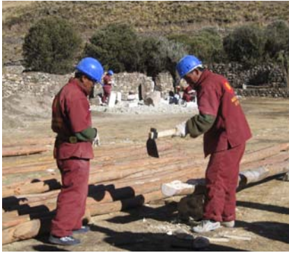
Figure 4: Local residents trained by AECID working on scaffolding for the church in Sibayo.
