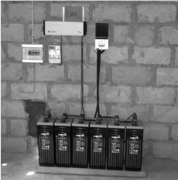
PICTURE 5. INTERIOR EQUIPMENT OF THE TECHNICAL ROOM. FOURDOU.
