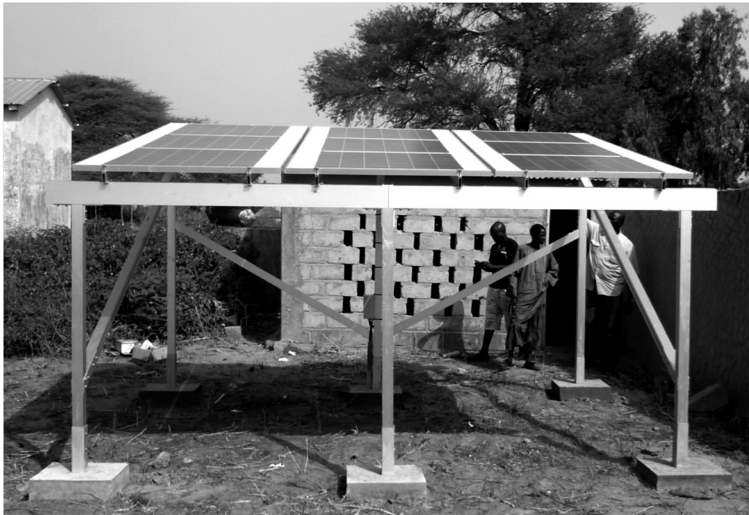
PICTURE 4. PV INSTALLATION AND TECHNICAL ROOM. FORDOU.
