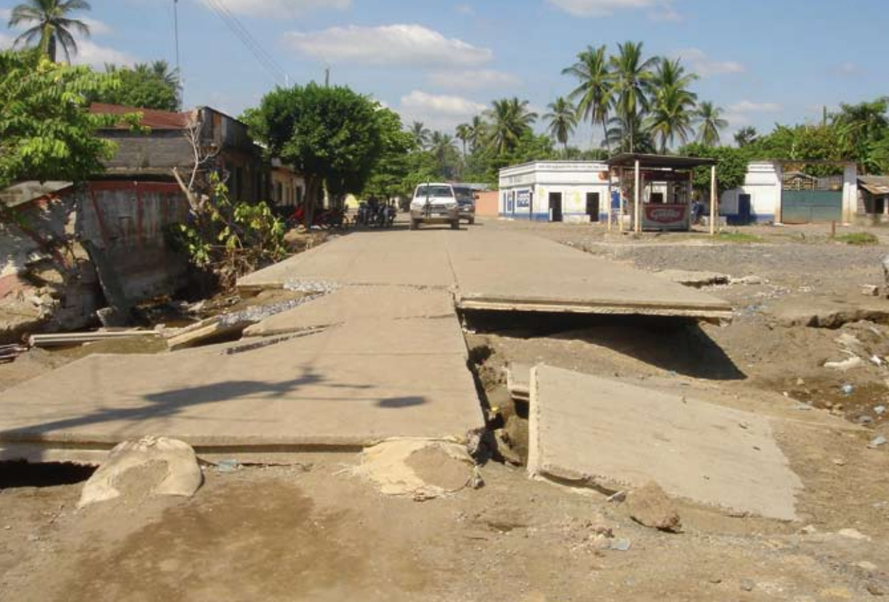
Infrastructure destroyed in Central America during the hurricane season. Source: USAID
